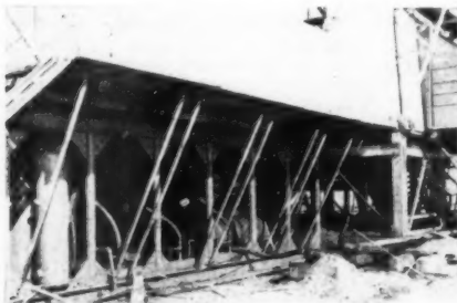
DUAL PURPOSE CATWALKS. —These catwalks on Rowan Drilling Co. rig in eastern New Mexico not only provide walkway for crew, but support engine-house wall. Note diagonal supports.
